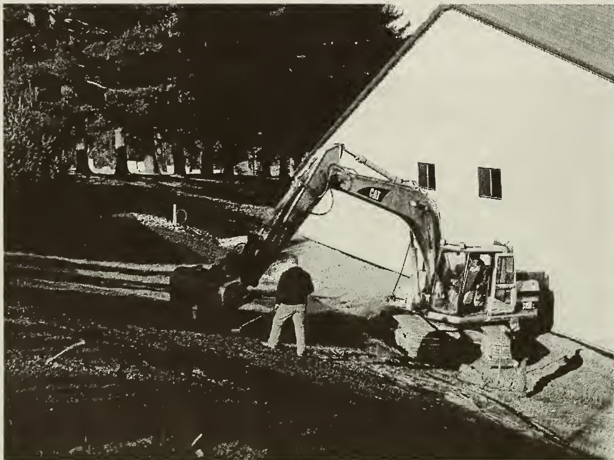
November 19, 2004. Final grading by Derby Mountain Construction of Lyme, NH (assisted by the Lyme Highway Department).
